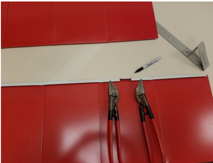
Use sheet metal snips to cut the seam at the marks to create a channel as wide as the snow hook 5066 West Amelia Earhart Drive - Salt Lake City, UT 84116
