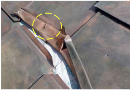
Roof system failure due to poor craftsmanship, design and implementation.
