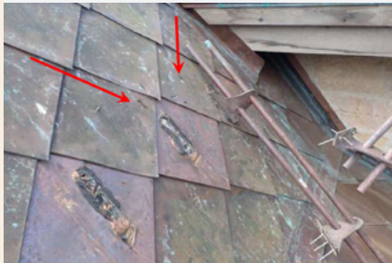
Poorly designed, placed, and installed snow fence resulting in failure all around.
