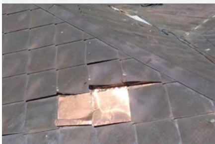
When even your replacements are failing, it's time to call us!
