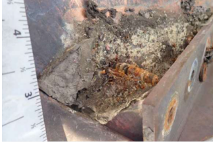
Withdrawn and fractured fasteners in galvanically dissimilar materials with extended exposure to water create massive corrosion.
