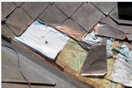
Under-engineered shingles are no match for weather.
